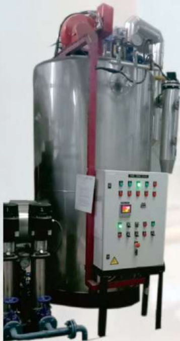
Vertical Steam Boiler
